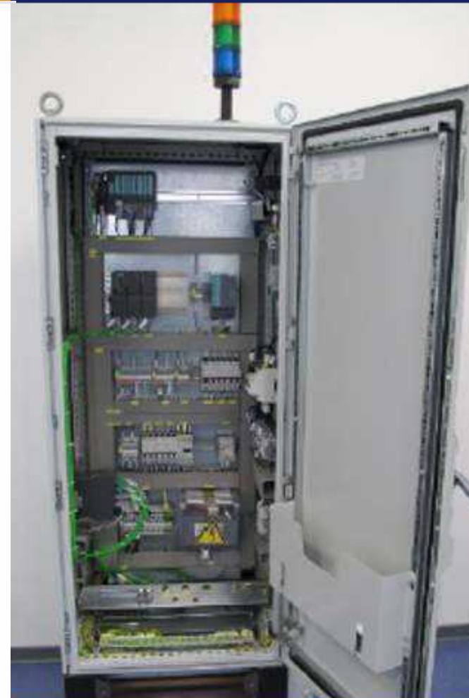
Cabinet, wiring, assembly
